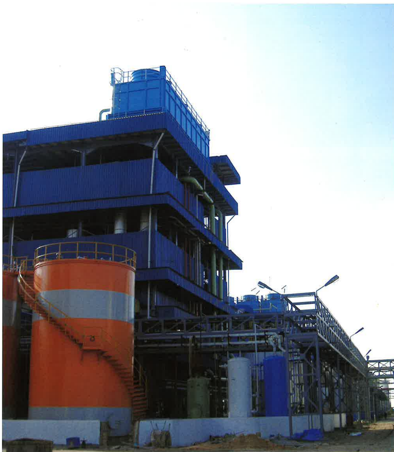
Overview of a 200 TPD Multi-Feedstock Biodiesel Plant in Indonesia.
