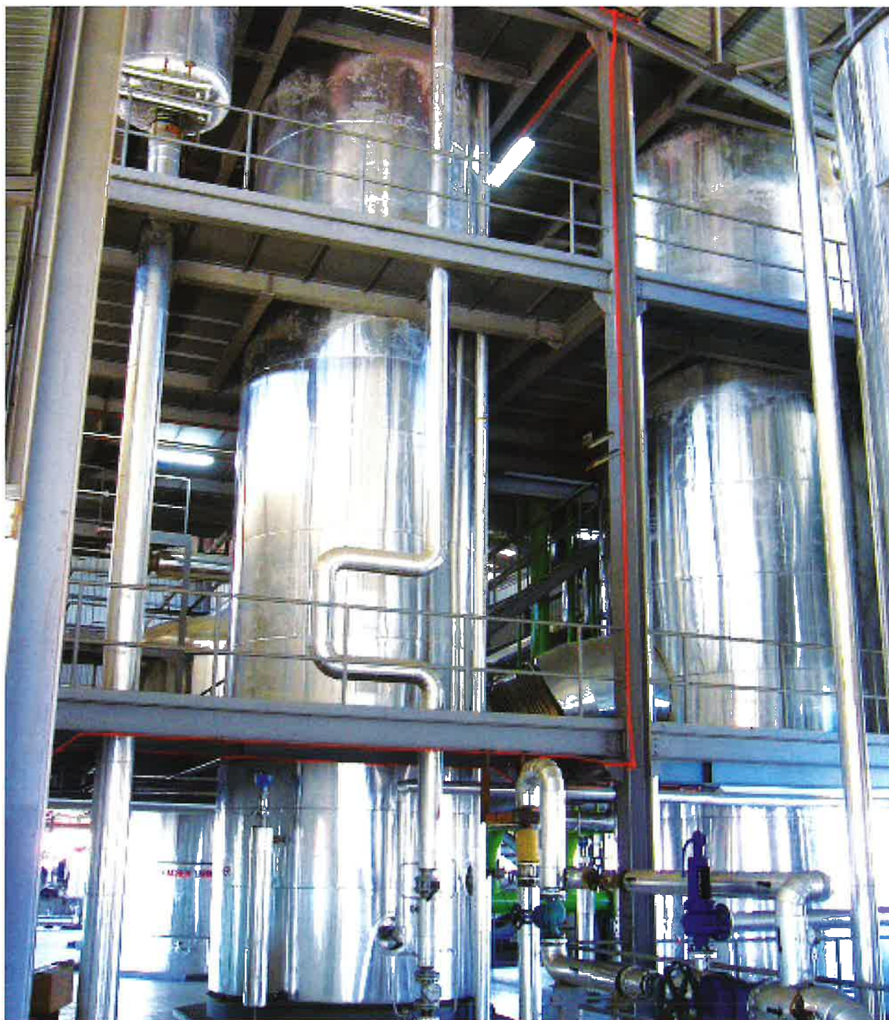
Deodoriser in a 1,500TPD Physical Refining Plant in Sabah, Malaysia.
